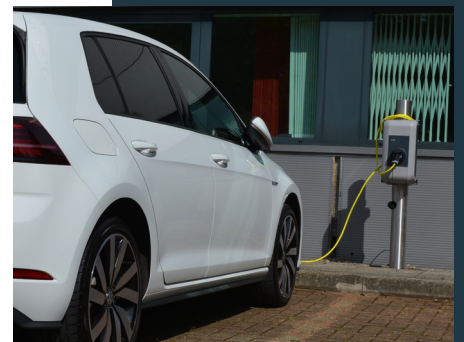
EV chargers available for customer use
